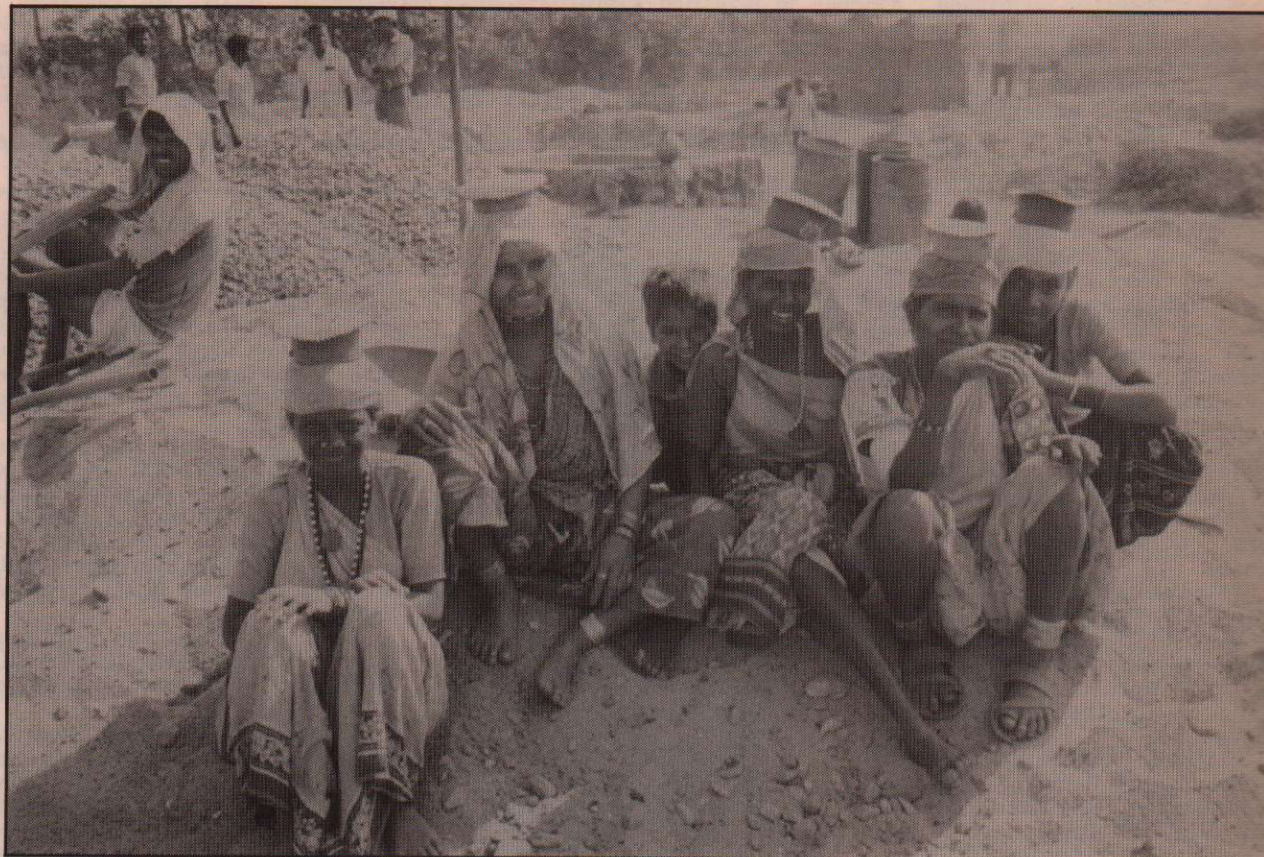
The heavy lifting squad waiting for the concrete to arrive for a bridge on the new railway
