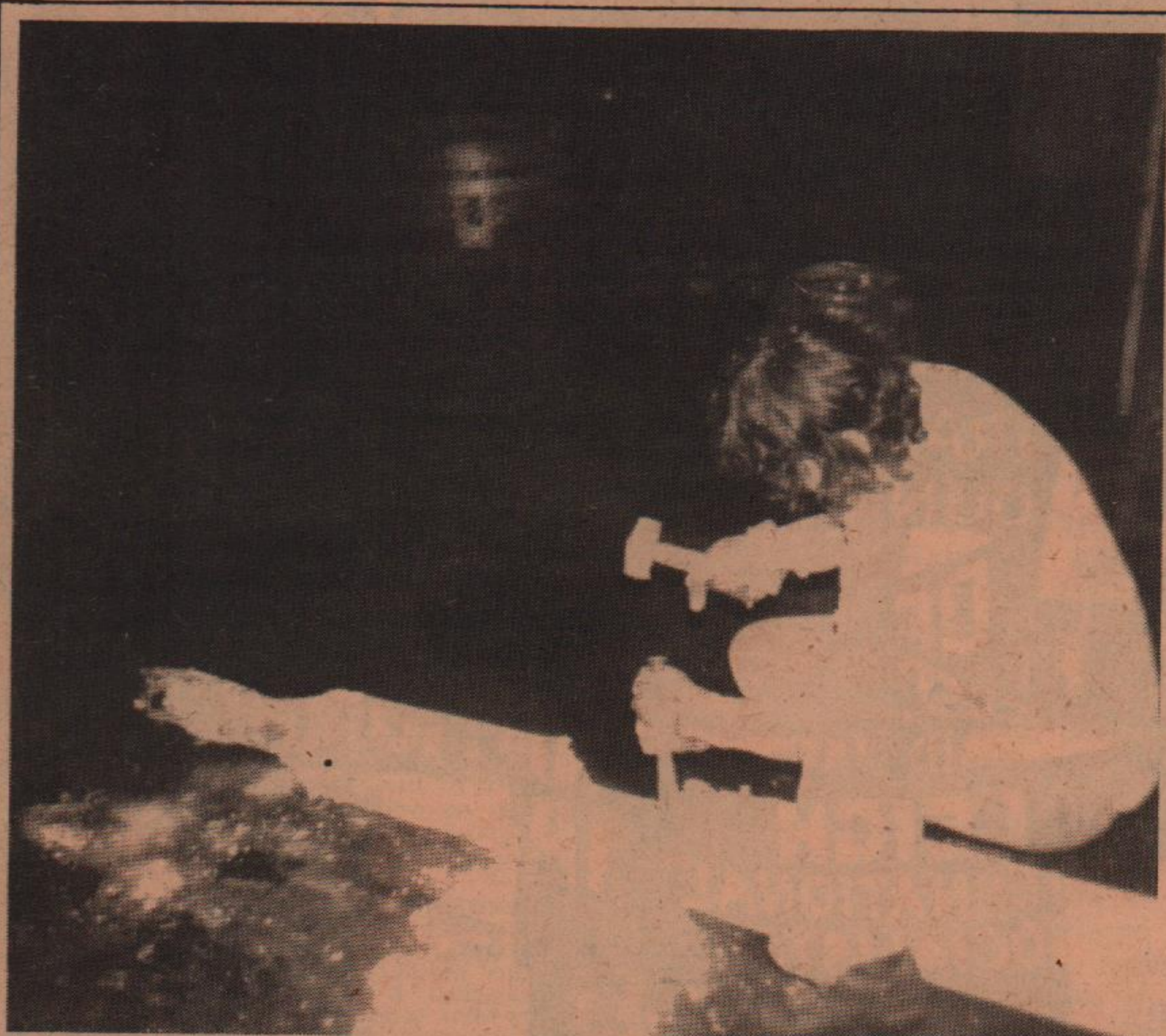
Asbestos being removed: unprotected worker, unprotected beer
