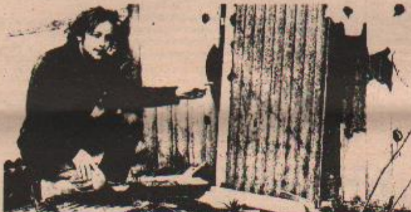
One of the asbestos panels broken when police and 'bailiffs' stormed Bason's last Friday.
